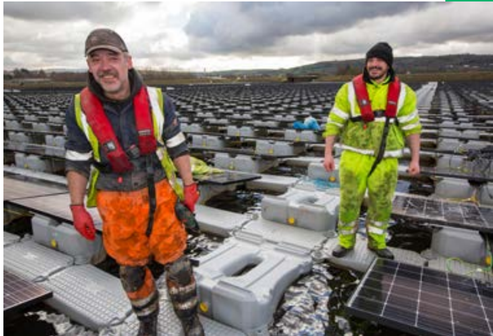
The new floating solar farm being grid connected on Godley Reservoir in Hyde, Manchester
